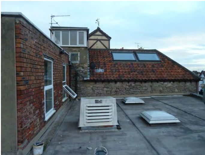
Plate 9. The front flat roof, rear 1 st floor section and relationship with the adjoining 'Ye Olde Cottage'.
