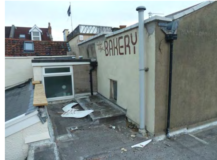
Plate 11. The rear elevation and boundary window on the side of 'Ye Olde Cottage'.
